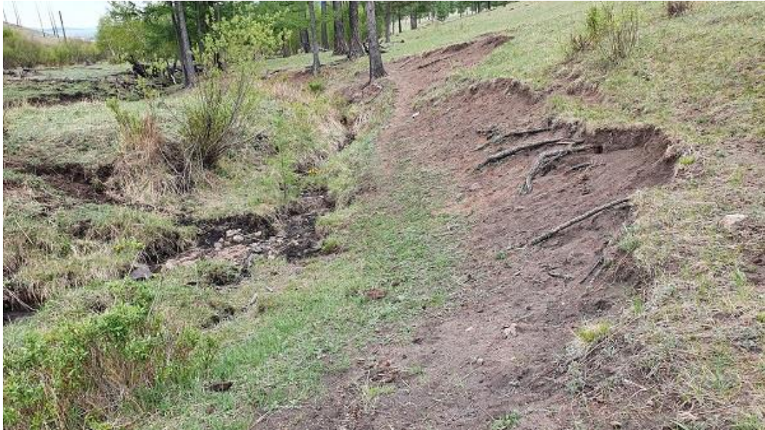
Figure 21: Slope erosion and loss of top-soil
